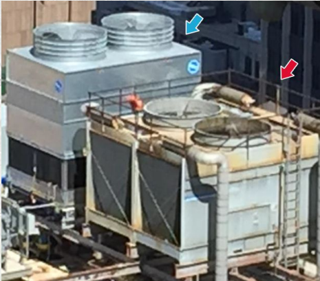
CDC - Photos of Cooling Towers
