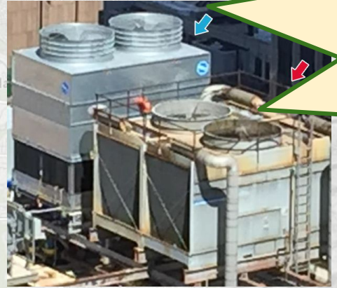
CDC - Photos of Cooling Towers
